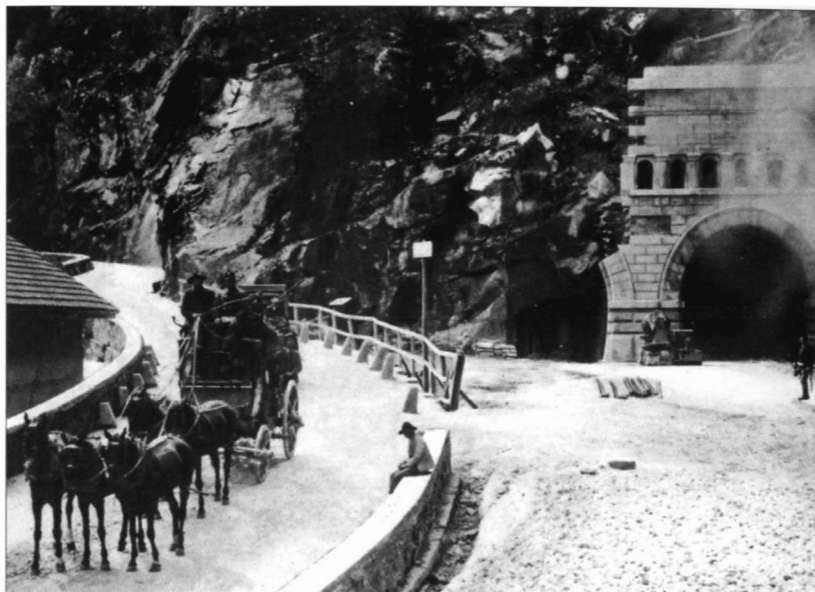
133. Simplon Tunnel, south portal during construction: right Tunnel 1, left entrance to parallel gallery. ( Gesellschaft für Ingenieurbaukunst, Zürich )
